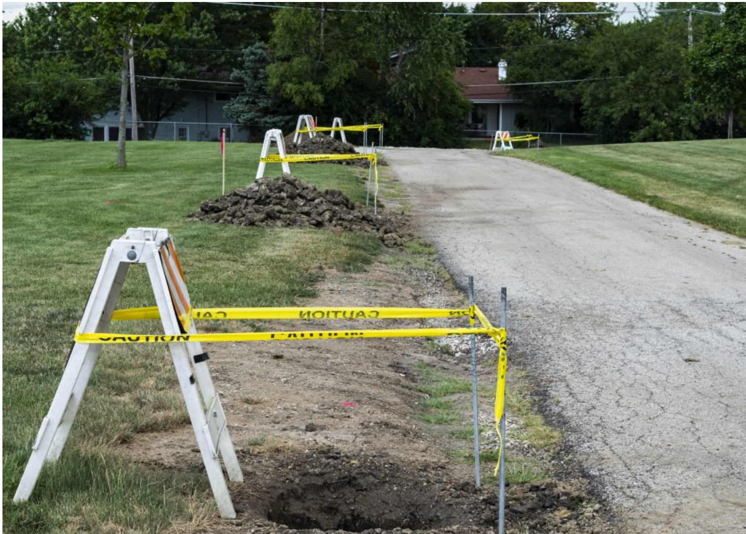
Crews dug out post holes for the installation of new safety lights between the fields at Hoffman Estates High School.
