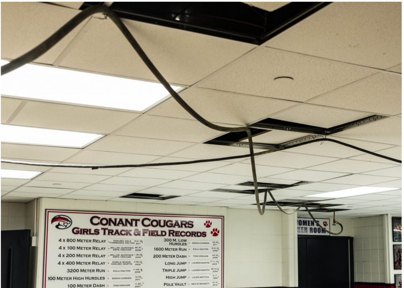
Temporary water lines span the ceilings of James B. Conant High School during construction on the school's bathrooms.
