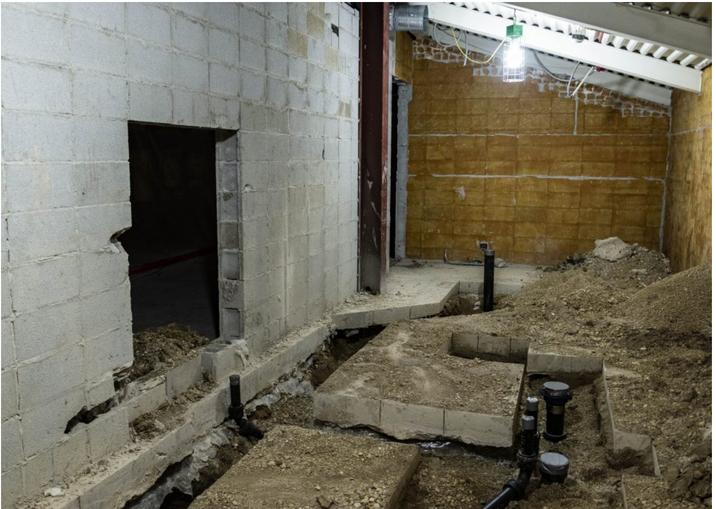
A bathroom at James B. Conant High School which has been torn down in preparation for a complete overhaul.
