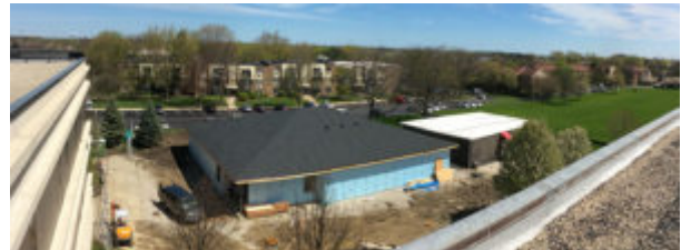
The Adult Transitions Program (ATP) North building, which is being constructed on the northeast side of Palatine High School, will be completed in August and ready for the first day of school.
