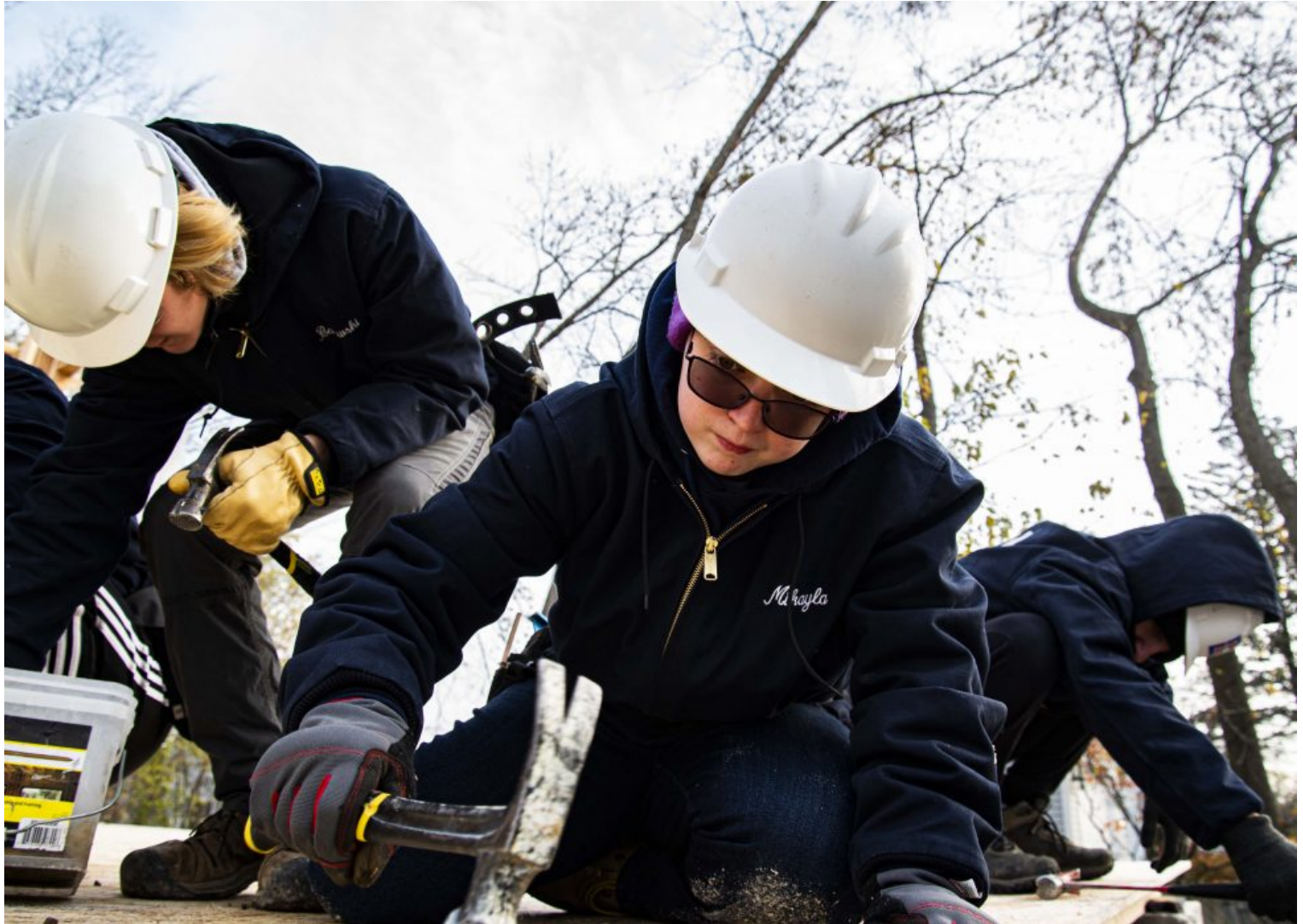
Students in William Fremd High School's Building Construction program work on a wall at the construction site in Palatine, Illinois, November 16, 2021.
